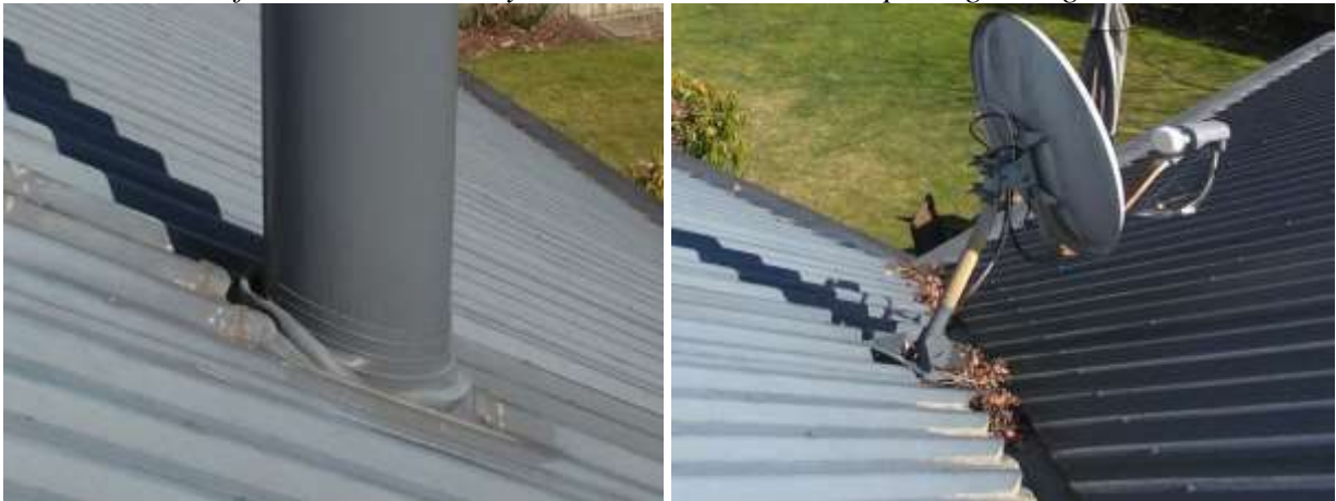
Good flashing to the chimney but will not comply for a replacement fire. more leaves in the valleys gutters
