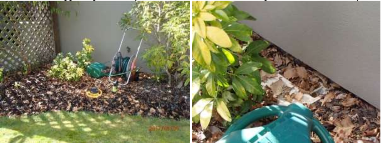
Garden levels are too high and this hidden gully is filling with leaves.
