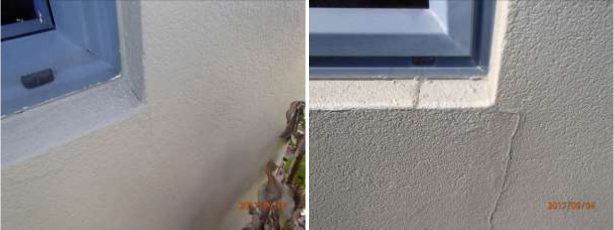
Some cracks have not been touched and some are very untidily patched
