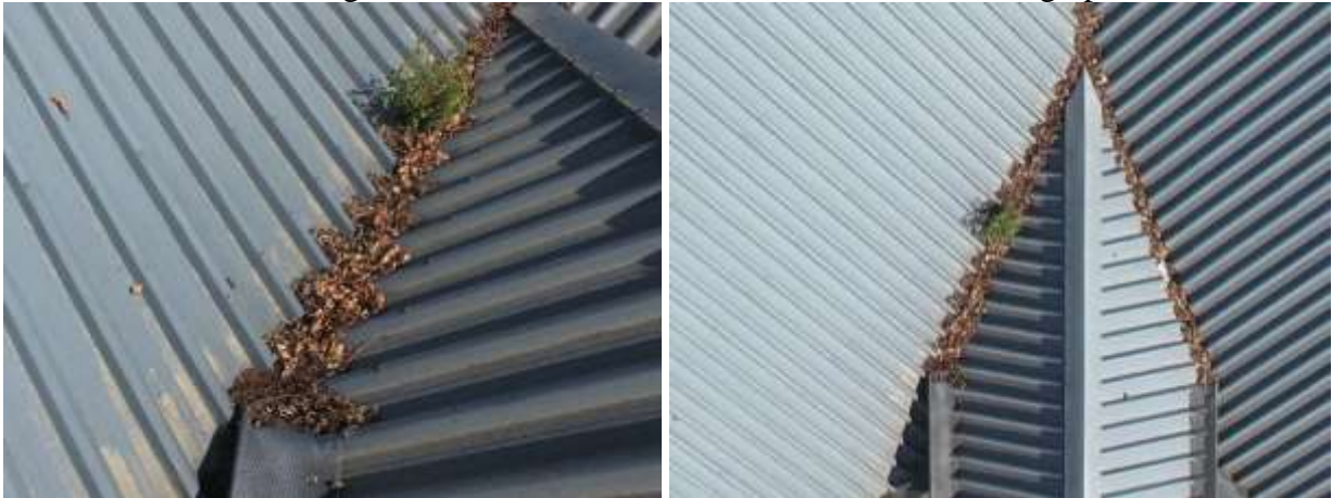
There are a lot of leaves in the valleys over the entrance and a plant growing
