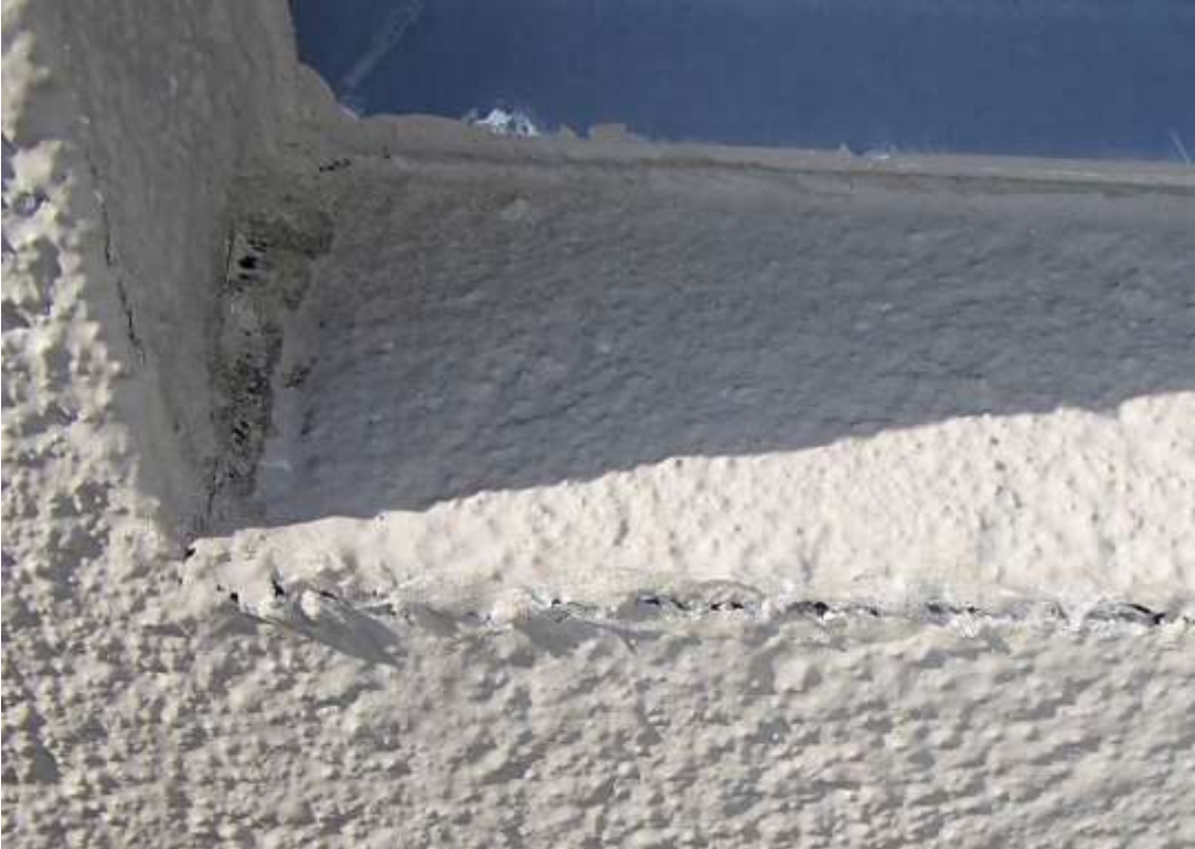
A lot of the sill flashings along this side and NE are lifting and need to be replaced.
